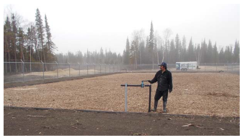
MCN's wastewater treatment plant operator Clarence Cook closes a valve used to expel condensation collected in the SAGR's aeration system over winter. PHOTO: LLOYD VASQUEZ, NEXOM
